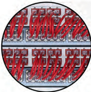
Direct Switch Patching with 8-inch Patch Cords
