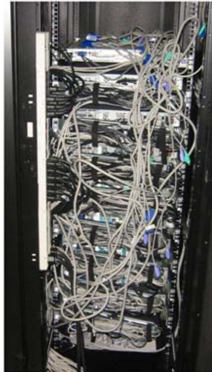
Figure 4. Poor in-cabinet cable management practices introduce clutter and choke points in the exhaust area that limit cooling system effectiveness.
