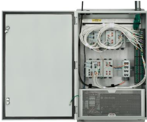
Figure 3. Integrated Network Zone systems from Panduit can offer 75% reduction in time to deploy. 1
