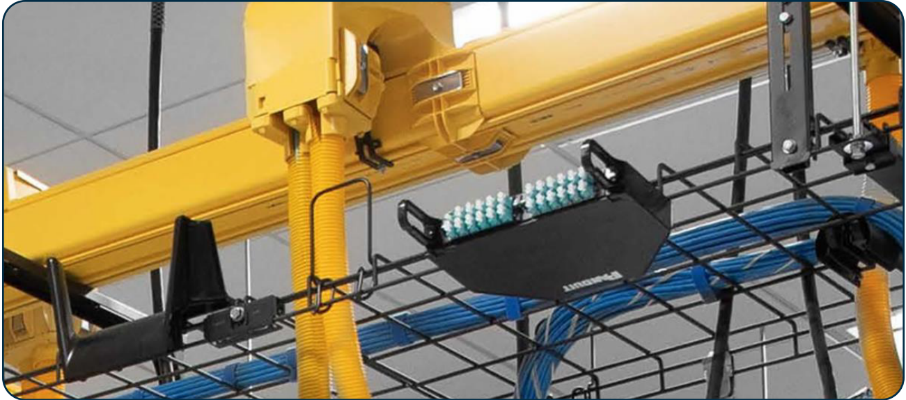
Figure 3. Equipment and telecom room fiber and copper pathways
