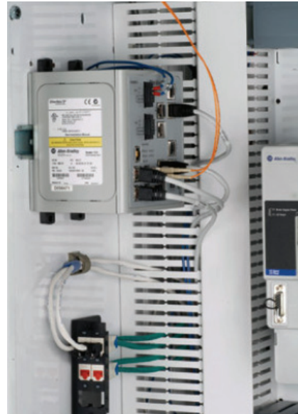
Figure 2.8-1. Ethernet Switch and Panduit Patch Panel mounted on Side Plane with PANDUIT PanelMax™ Corner Duct
