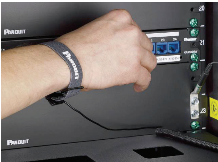
Figure 4.3-12. ESD wrist straps and ports enhance equipment protection.
