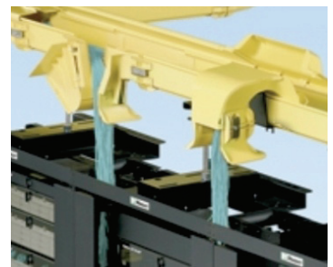
Figure 4.5-4. Example installation of FiberRunner® overhead pathway showing transition to 4-post racks. Cable is 12-fiber jacketed ribbon interconnect.
