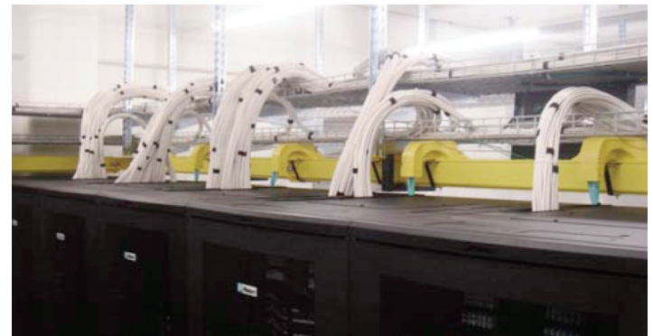
Figure 4.5-5. Example installation of FiberRunner® overhead pathway to PANDUIT® NetAccess™ cabinets. Cable is 12-fiber trunk. Note copper cabling installed in wire basket above FiberRunner® pathway system.
