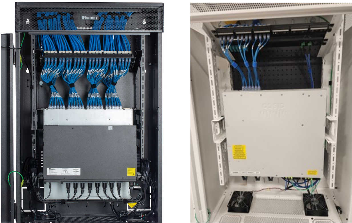
Figure 39. Cisco Catalyst 9300 deployed in Panduit TrueEdge
