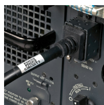
Electrical Infrastructure Labeling
