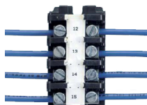
Terminal Block Labeling
