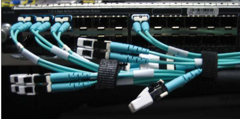
Figure 1. Fiber Switch Blade not utilizing all LC connectors on the hydra cable
